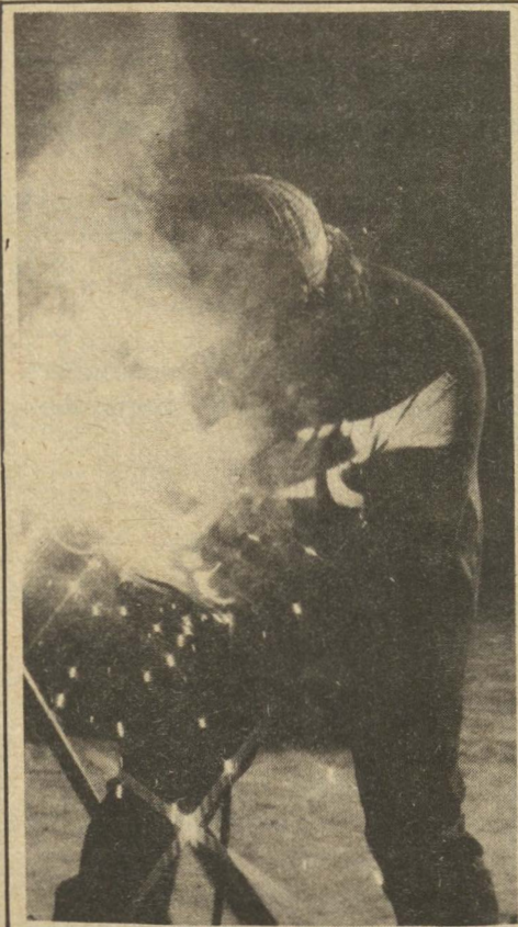
Like a character out of "Star Wars," a welder puts the finishing touch to his work.
