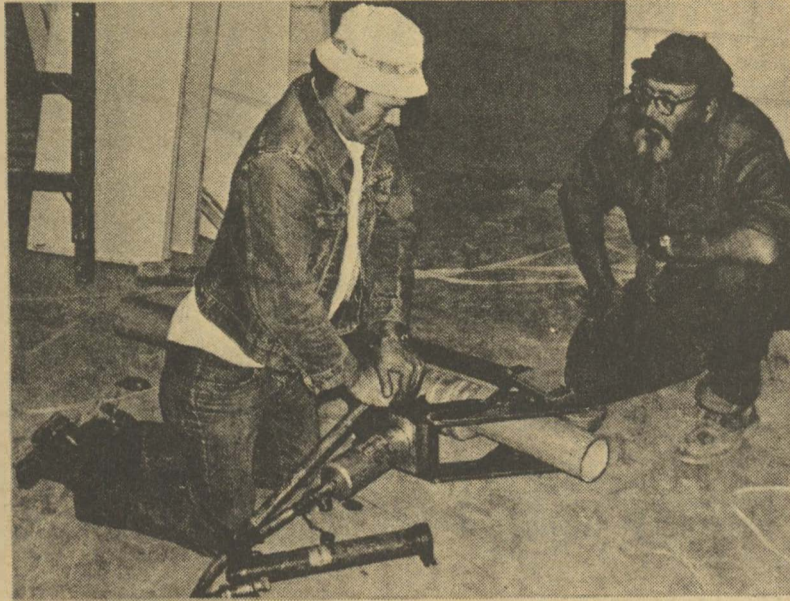
Workers prepare the site for the new computer center to be located in Towers Hall.
