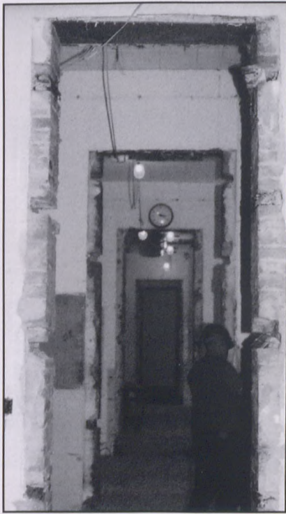
Towers looks rough now, but soon it will shine with a new luster! This is the first floor toward the front of the building.
