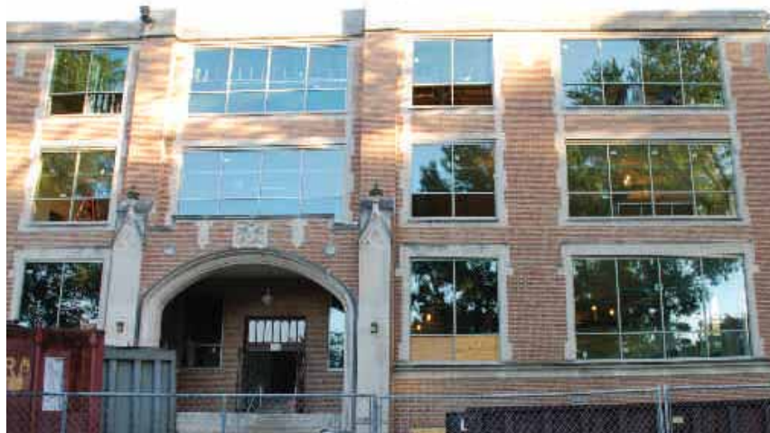
Campus trees reflect off newly installed window panes in McFadden Hall. The large panes have been installed into the original large window spaces, which have been opened back up after being mostly bricked in for several decades.
